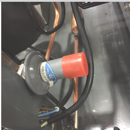
Hot gas Bypass Valve
